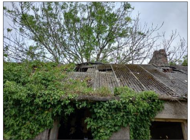
Plate A4. Large gaps in roof exterior of B5
