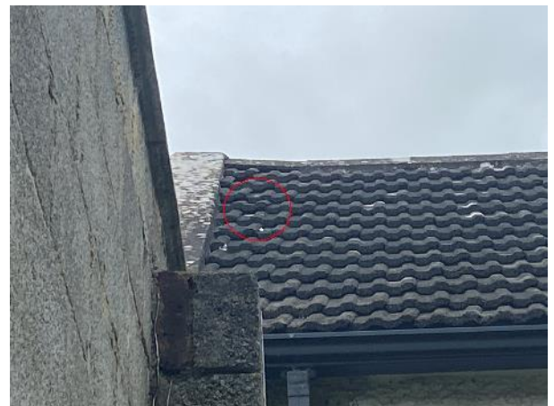
A12. Indicates identified bat emergence point at B6.
