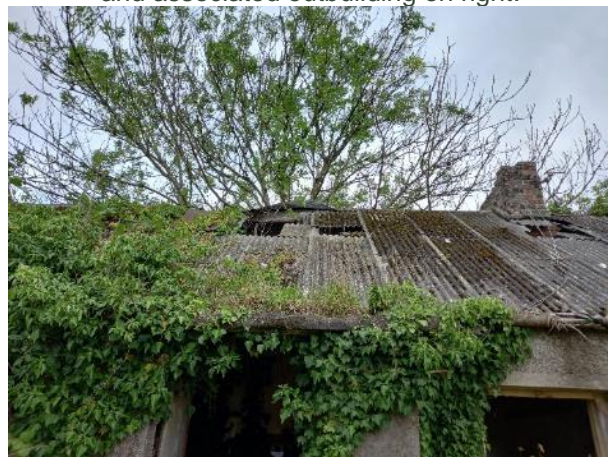
A4. Large gaps in roof exterior of B5.
