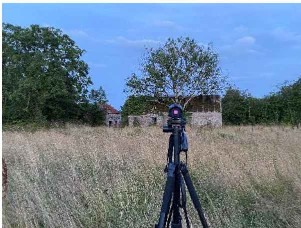
A3. Northern elevation of B5 viewed showing view of thermal imaging camera.
